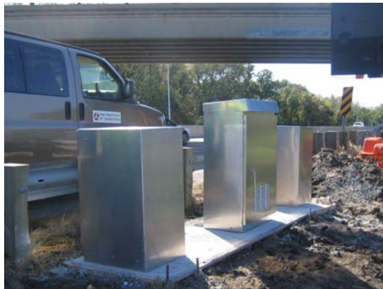
Three cabinets house the two AxleLight sensors (in the outside cabinets), with the ADR-3000 Plus unit, the power panel, and the batteries housed in the center cabinet
